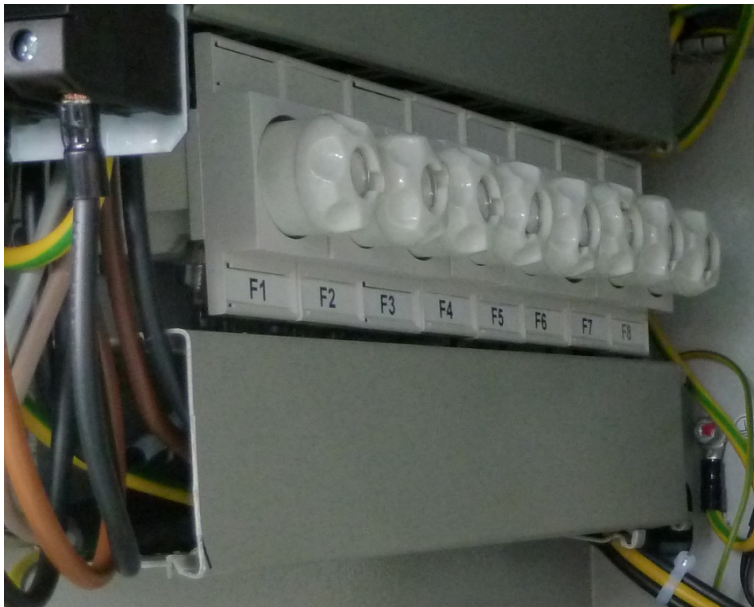
Figure 43: Circuit breaker of the NS distribution in the control unit
